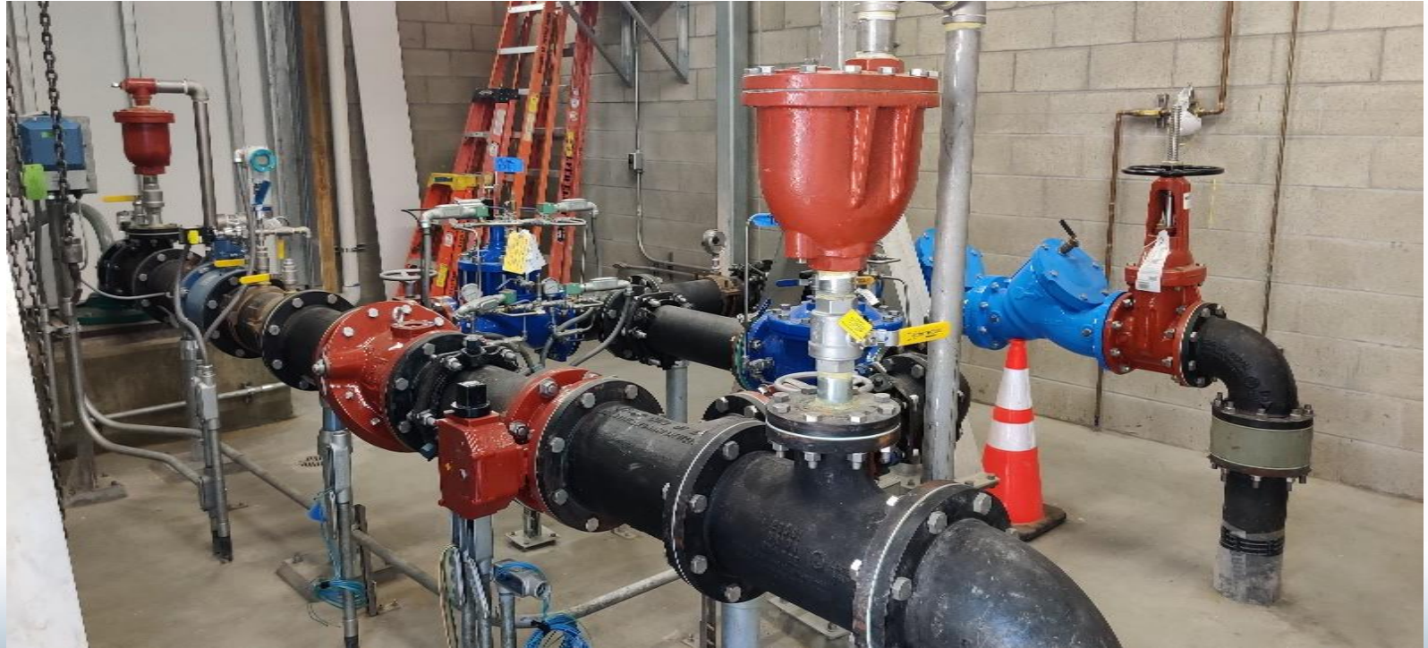
Interior Piping with Alternative Valves
